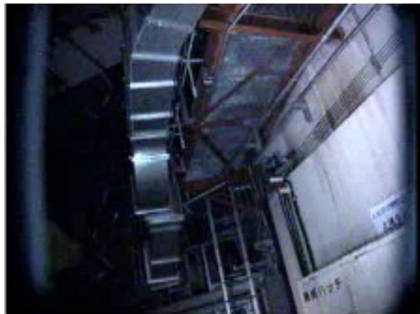
Check of the leakage from the electrical penetration
