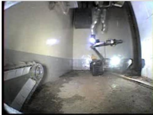
Nearby the entrance of SHC pump room
