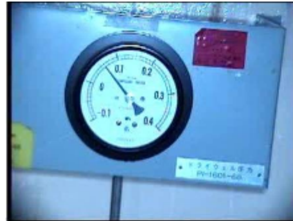
Observation of the pressure gauge of the primary containment vessel
