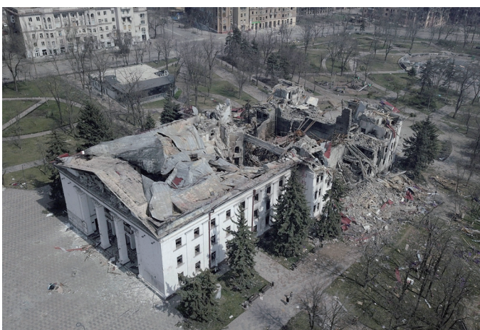
A view shows the building of a theatre destroyed in the course of Ukraine-Russia conflict in the southern port city of Mariupol, Ukraine April 10, 2022. Picture taken with a drone. REUTERS/Pavel Klimov (Ukraine)
